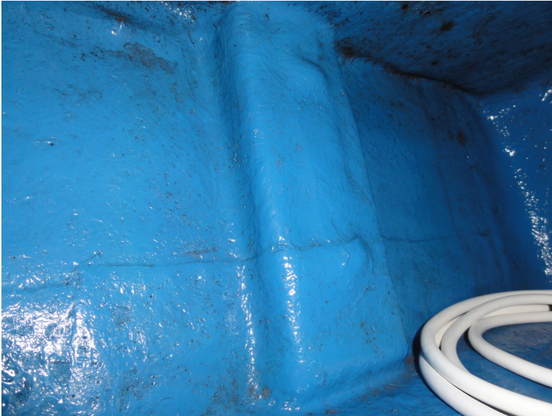
Original chainplate assembly glassed over in a cupboard (fwd lower shroud)
